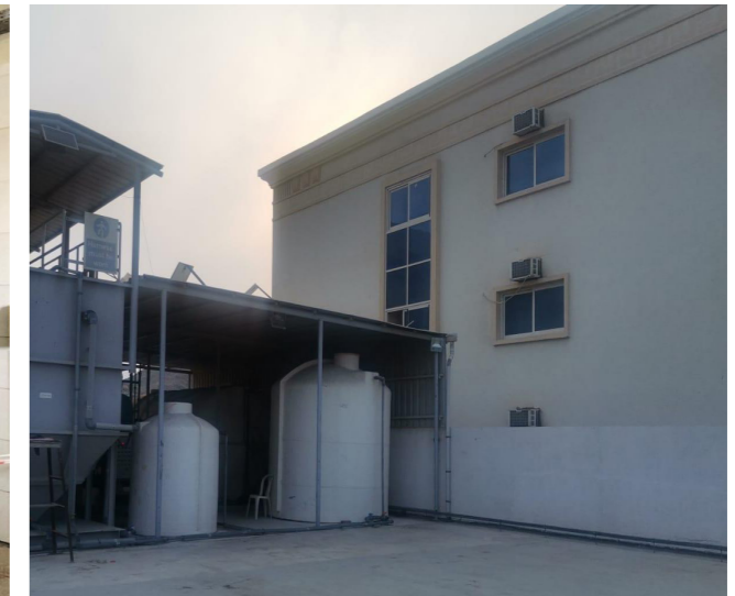
Sewage Treatment Plant at Fujairah Accommodation
